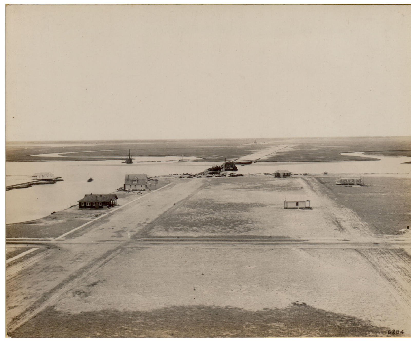
Circa 1910 - A striking view of 96th Street under construction. Looking west we see the making of the Stone Harbor Boulevard linking Stone Harbor with the mainland. A draw bridge in the making over the Great Channel destined for an official opening on July 3, 1911 with important dredging equipment in the background.
